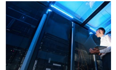
EQUINIX, PA10, Paris Data Halls: 3,750m 2 IT Power: 4.7MW
