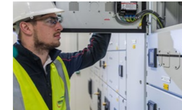
VIRTUS Data Centres, LONDON4, Slough Data Halls: 10,600m 2 IT Power: 27MW
